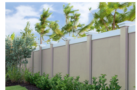
8' privacy wall of pre-cast, painted concrete along buffer (full buffer not shown)
