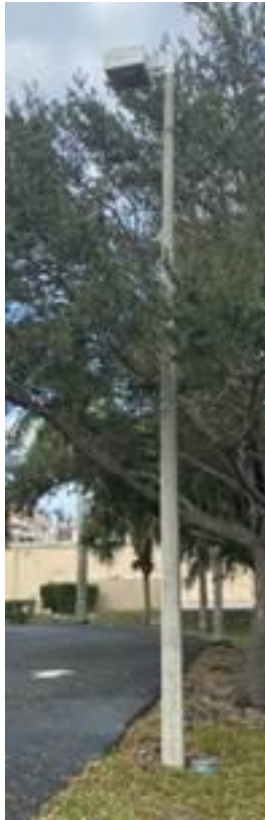
Existing Light Pole
