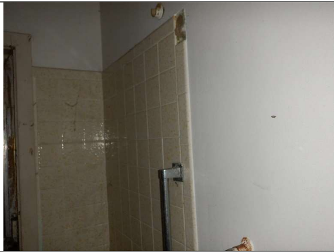
HM-R: Shower Tile/Grout/ Mastic, White
