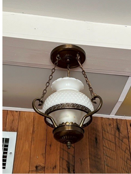
Item 15 - Light Fixture
