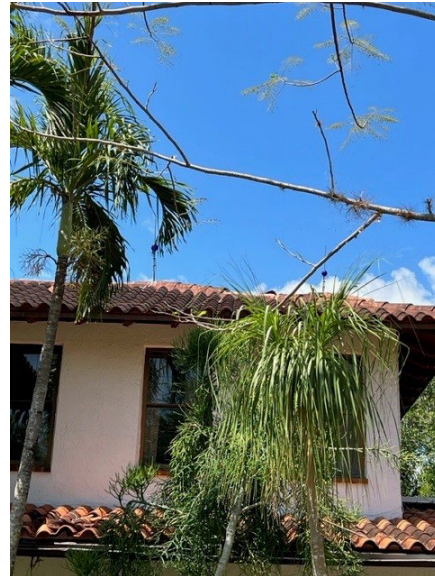
Item 4 – Two Lightning Rods
