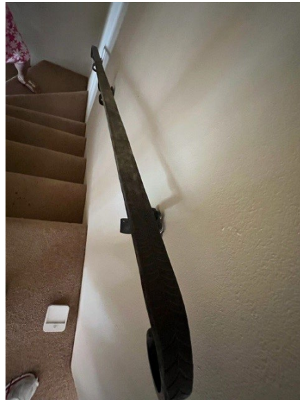
Item 8 – Stair Handrail
