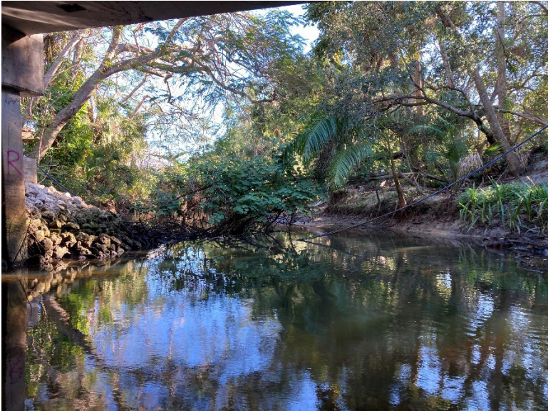
Small tree and downed communications cable on upstream side of Sandy Lane bridge
