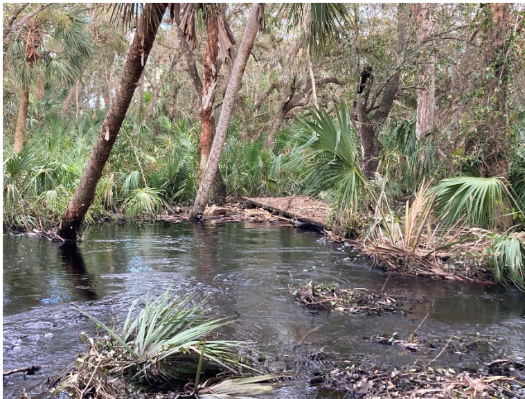
Flow restrictions by trapped limbs and debris at the old wooden walk bridge on the River Oaks property. View is looking east from the west bank.
